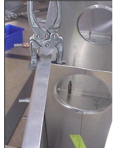
Clamp the Rear Tail Frame to the Side Skin. Line up the Tail Frame with the predrilled holes.
