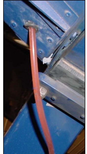
Location of grommet in cabin floor, see bottom left diagram on drawing 7-F-9
