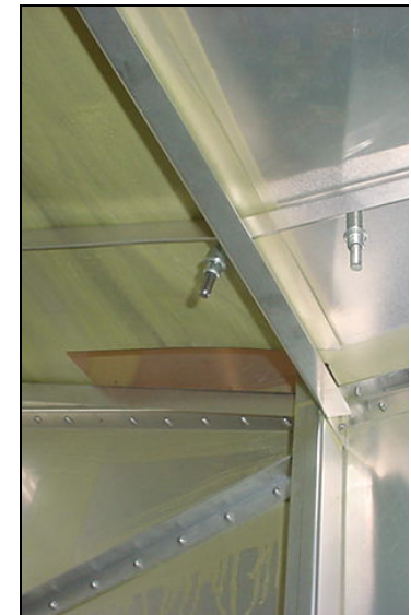
Photo of left side. 'L' angles on the front and aft side of the Zee Channel 7F8-10B
