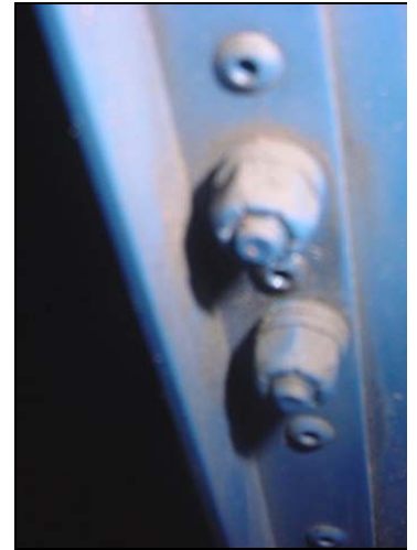
The bolts are through the Front Bottom Longeron 7F10-3
