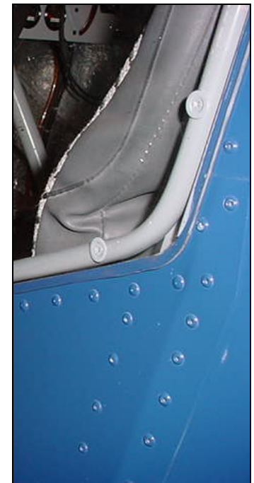
Detail bottom aft corner of left door on our demo: door overlap fuselage.
