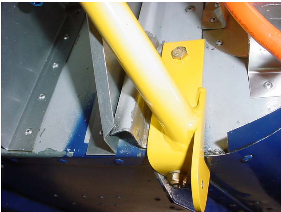
Left lower attachment COMMENT: Drill and cleco the engine mount to the firewall with pilot holes.
