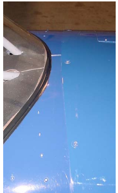
The cowl overlap on top of the fuselage skins that overhang past the firewall.
