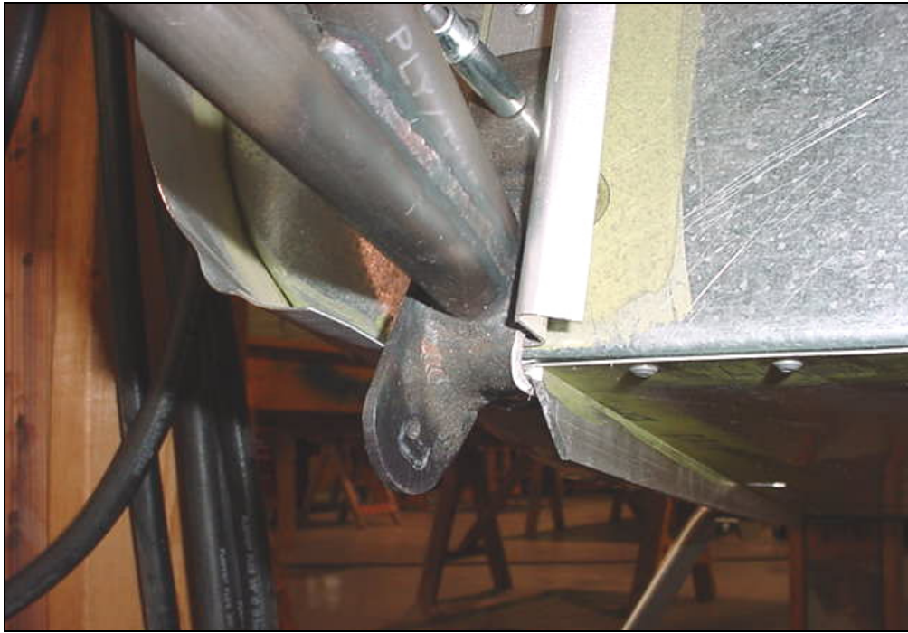
Bottom right engine mount attachment points to the firewall Check: That the Lower Bracket is not sitting on top of any rivets. 2 BOLTS AN3-5A Bolted through Firewall Stiffeners 7F7-5
