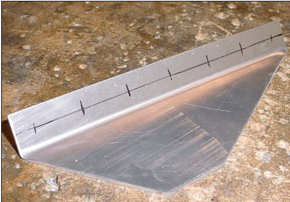
Front strut fitting doubler 7V8-1SP Layout the rivet line 9mm from the bottom edge. End holes are 10mm in from the ends.
